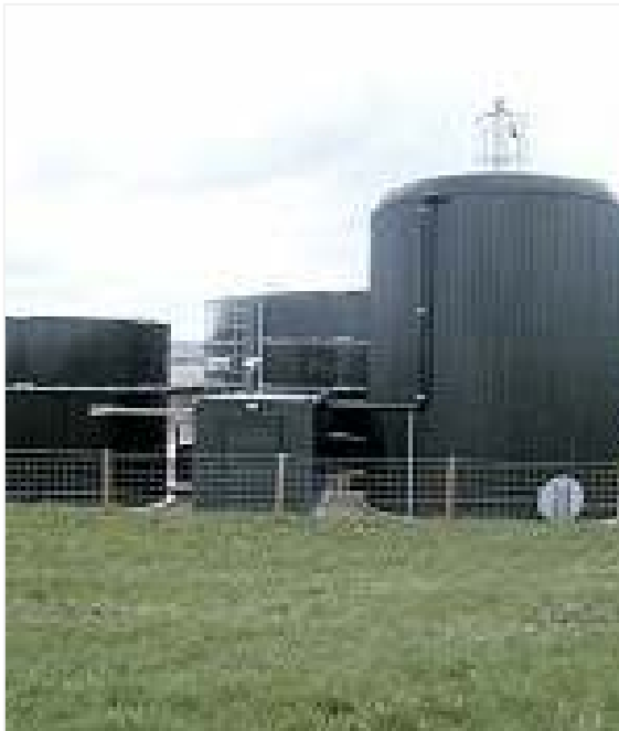
Figure 2-18. Anaerobic Digester (Biomass Energy Centre, 2015)
