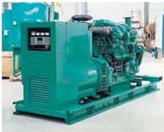
Figure 2-19. Reciprocating Engine (Madison Gas and Electric, 2015)
